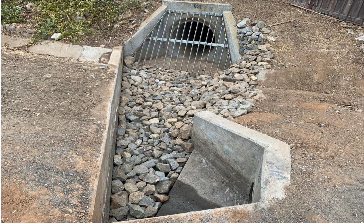
Photograph 17. Updated south view of concrete grated culvert where all three features convey flow.
