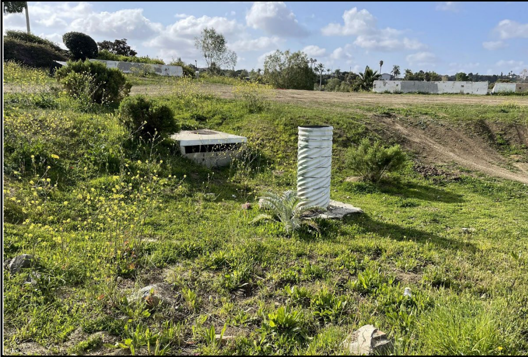
PHOTOGRAPH 4 Overview of Manufactured Drainage Area on Northern Terrace, Looking South
